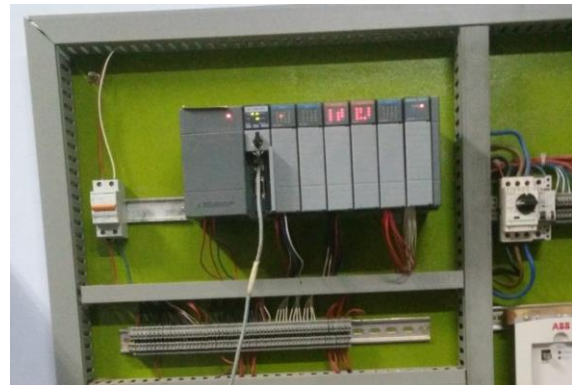
Gambar 2. 1 PLC (Programmable Logic Control) Allen Bradley SLC-500 di Area Crusher Sumber : PLIC
