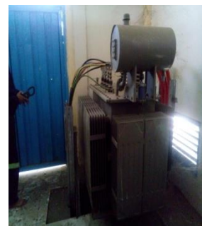
Gambar 3.2 Trafo Control Tuban 3
