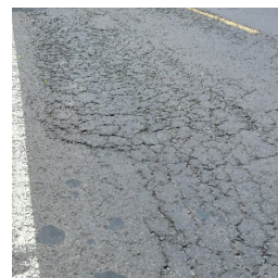
Retak Buaya (Cracking)
